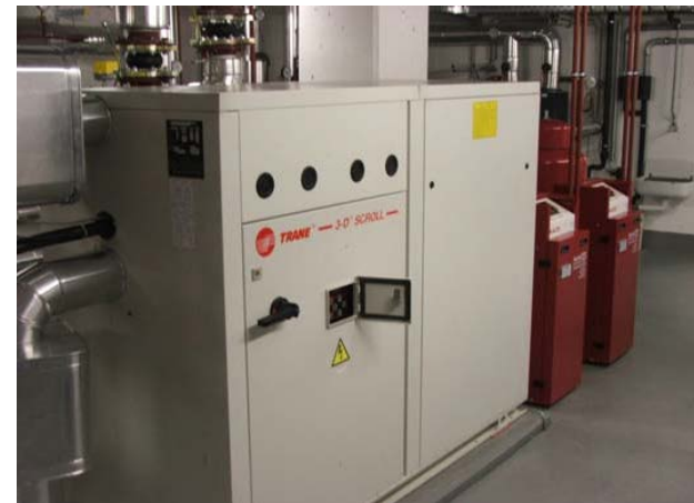
Heat pump MA30 sewage plant Blumental
